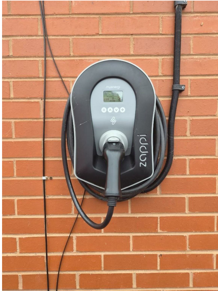
Car Recharging Point.
